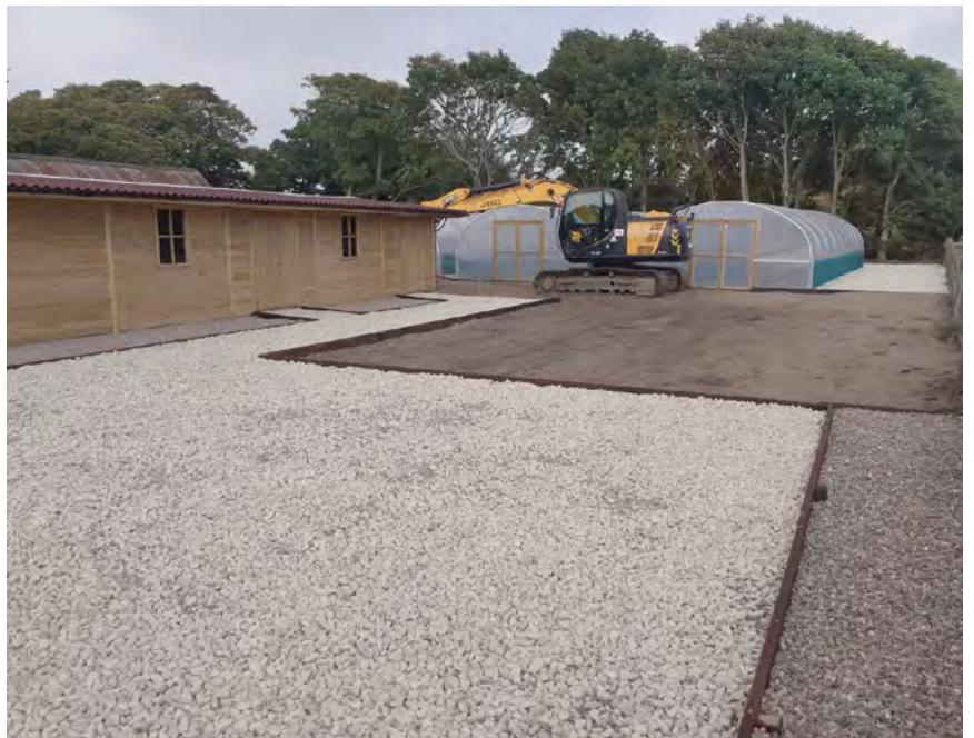
Wilder Humber new Seed Bank & Plant Propagation area construction, Lincolnshire Wildlife Trust, 2024.
